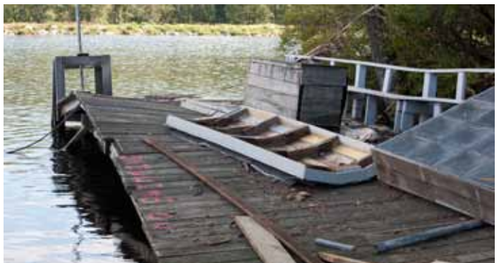
The swim dock after Hurricane Irene, 2011 - now in need of rebuilding
